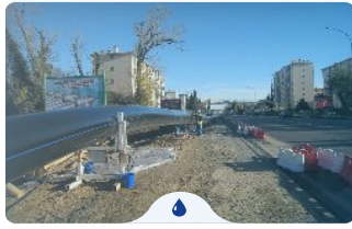
Drinking water supply
